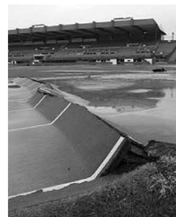
QEII damage by the 200m start area
